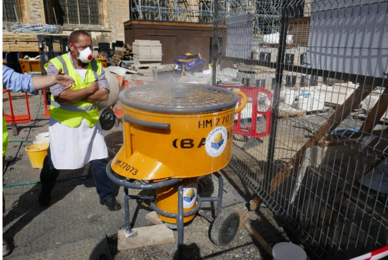
Photo 1 A mortar mill mixing “hot lime” mortar during conservation works at Canterbury Cathedral. Note steam from the sand slaking of quicklime.
