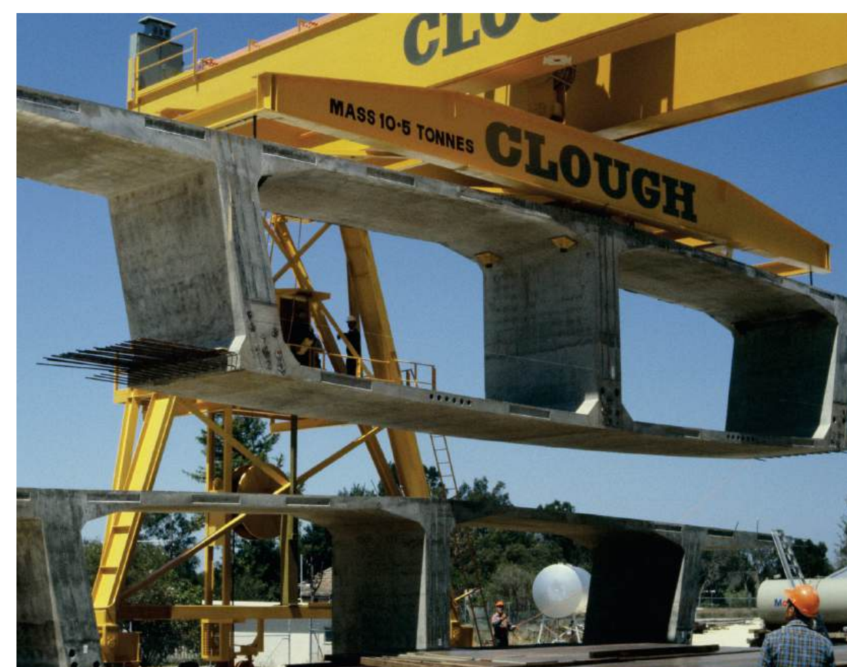
A 110 tonne unit for the 1982 Bridge
