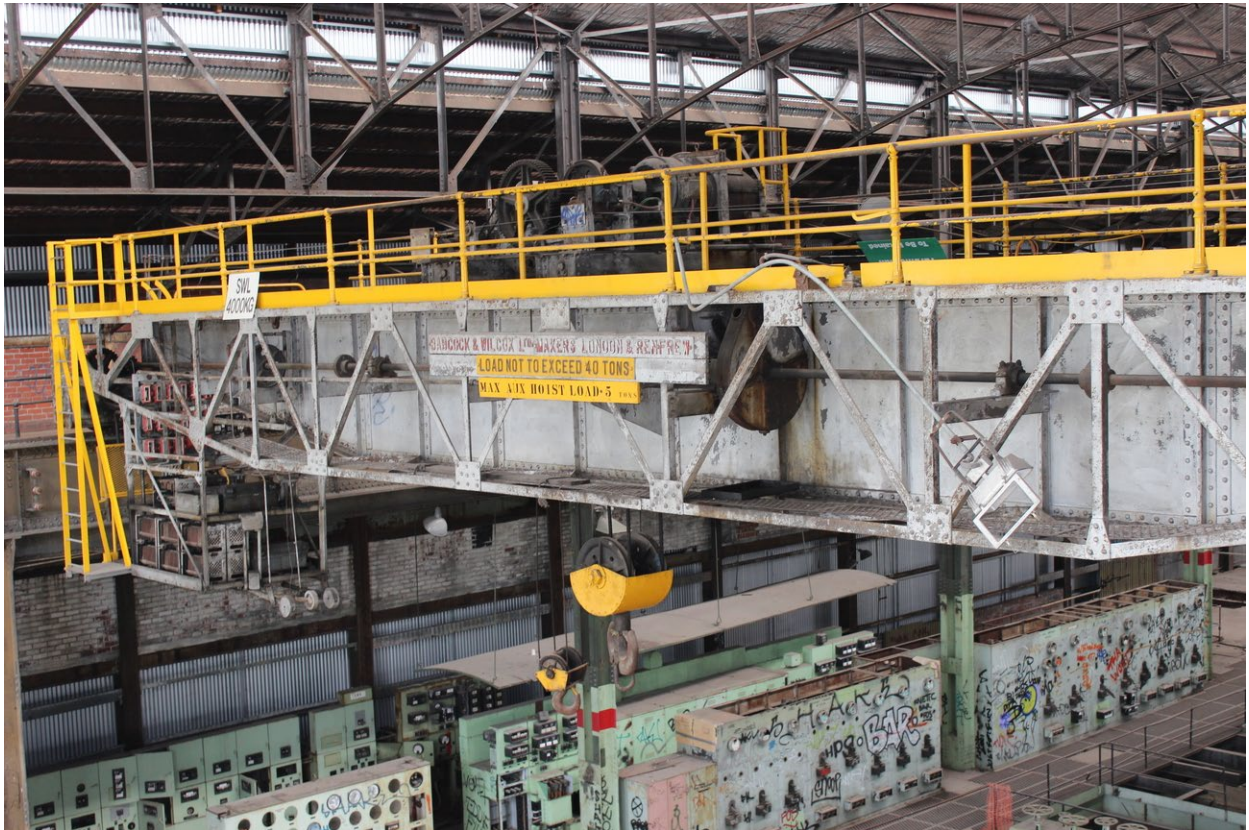
Figure 50: 40 Ton Gantry Main & 5 Ton Auxiliary Crane
