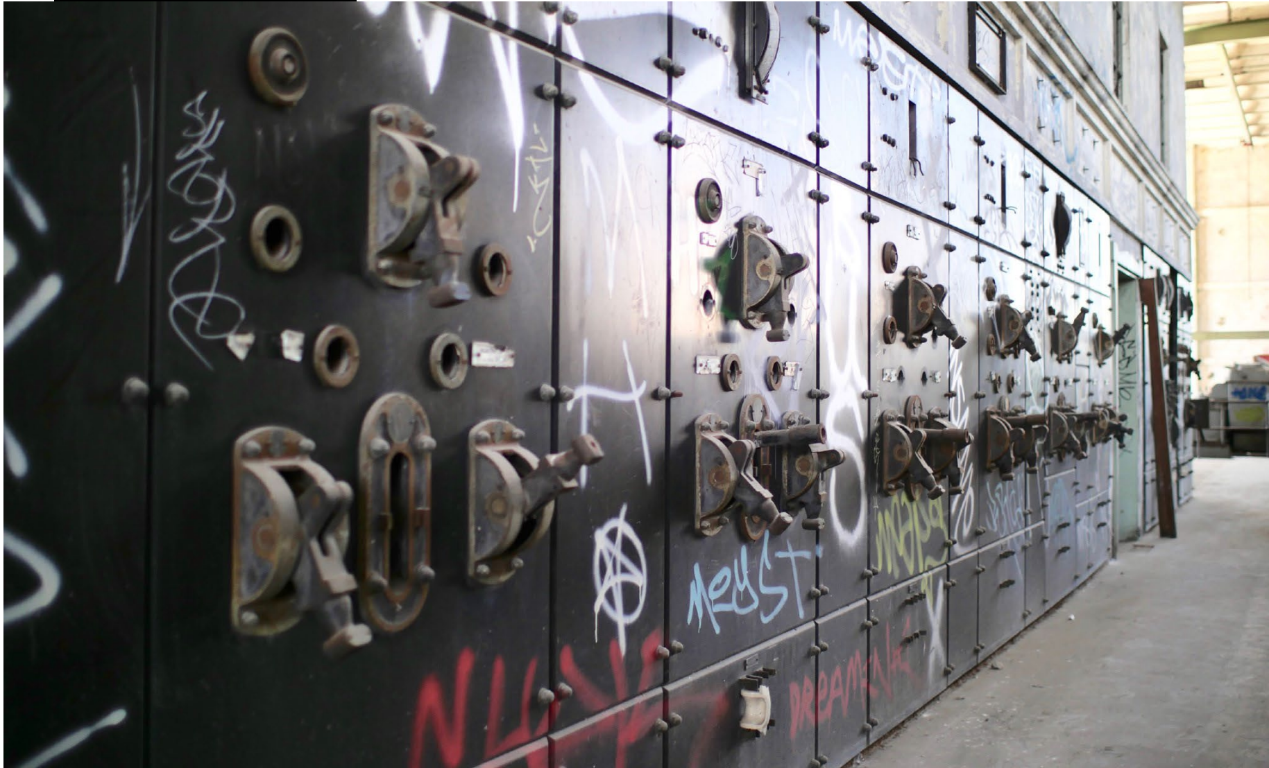
Figure 41: Original Slate Switch Boards form 1916
