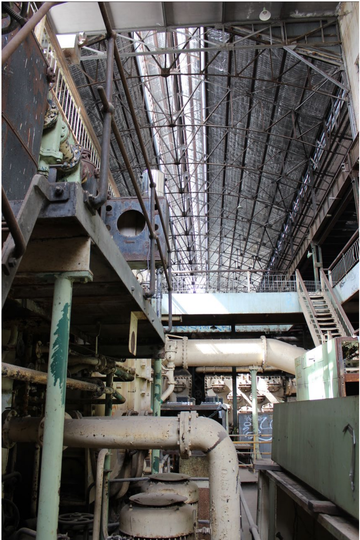
Figure 46: Condenser of Turboalternator No 5 viewed from beneath TA No 6
