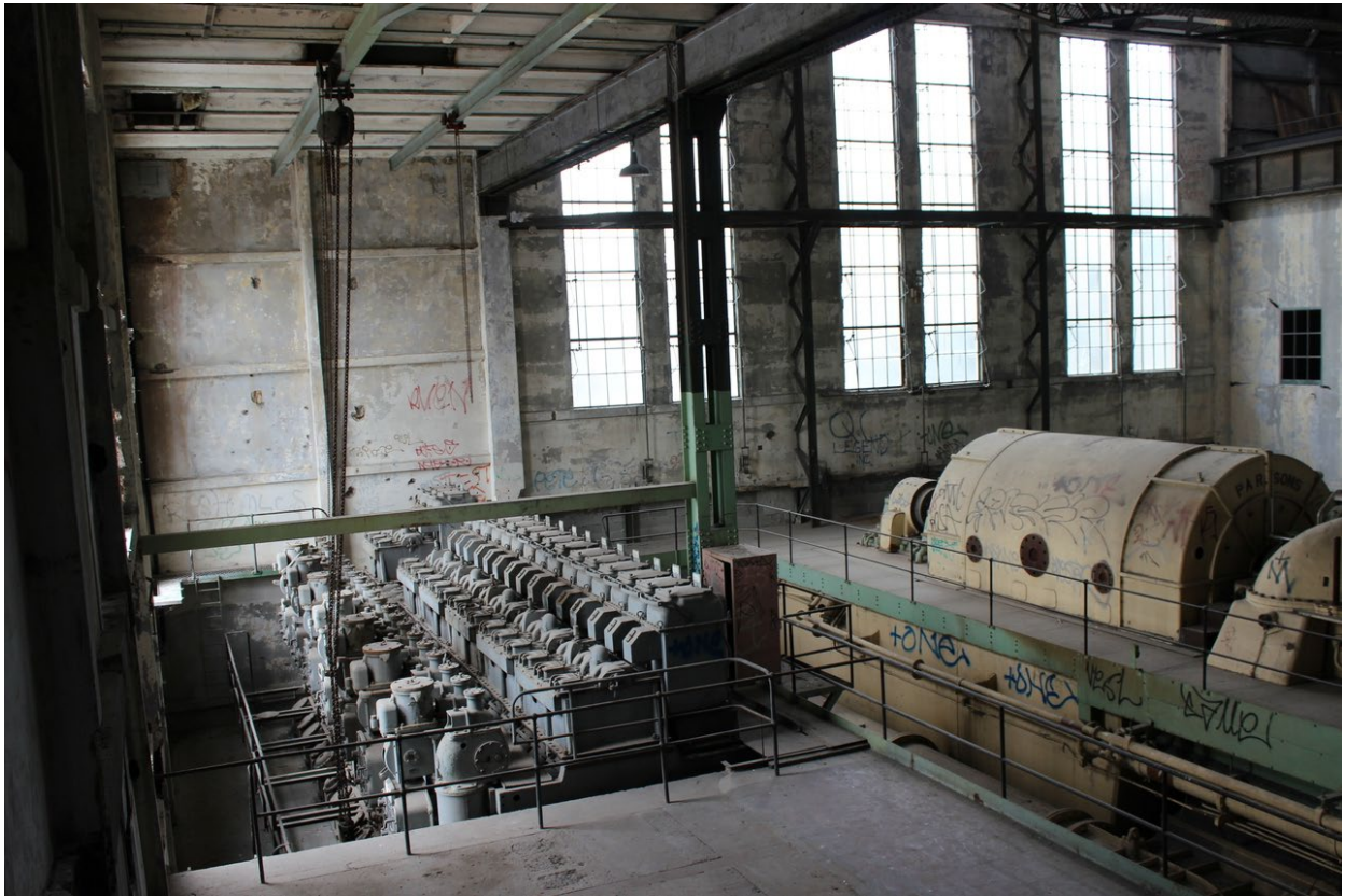
Figure 48: Turboalternator No 7 and associated 22, 000 V Switchgear
