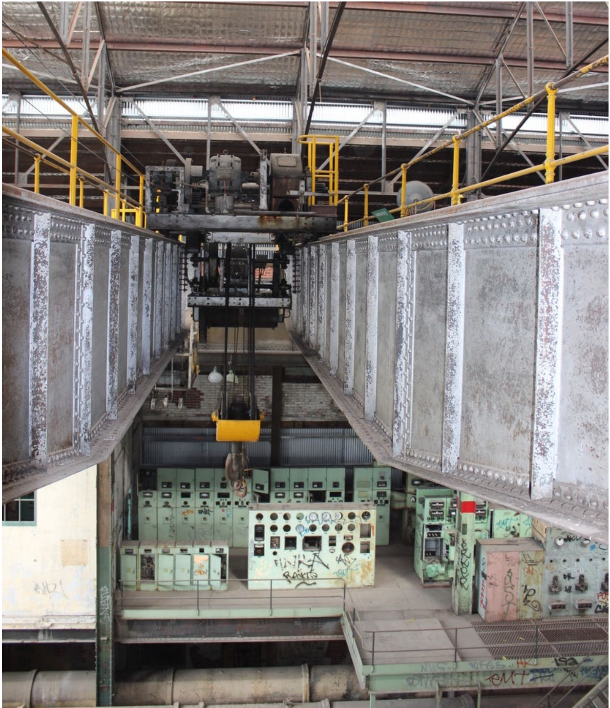
Figure 51: Gantry Crane Lifting Trolley
